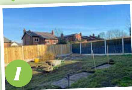
1 GROUND PREP BEGINS with removal of the old turf and patio – a blank canvas bonus is having less to debris to deal with!
