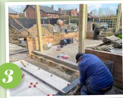
3 THE PERGOLA BASE, wooden uprights, timber beds and trellis screening go in, and tiles are laid for the patio. Phew!
