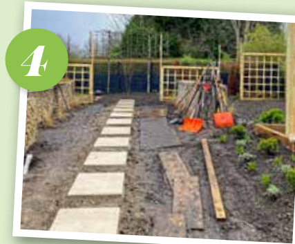
4 STEPPING STONES are laid in the centre of the garden, with pleached trees added for shade and screening.
