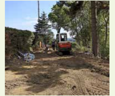
The hedge is tamed and the digger goes in to excavate the compacted, poor soil and level the area.
